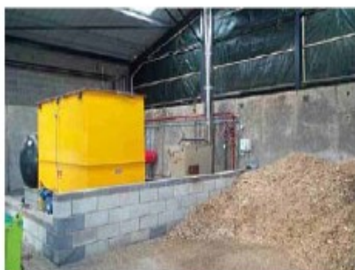
Figure 2. A Veto (80kW) wood chip boiler heating a farmhouse, two cottages, a café and business units
