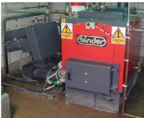
Figure 6. Binder (50kW) wood chip boiler meets 50% of large educational centre's hot water
