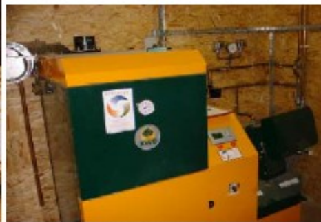
Figure 5. KWB (25kW) wood chip boiler heating an organic farm shop
